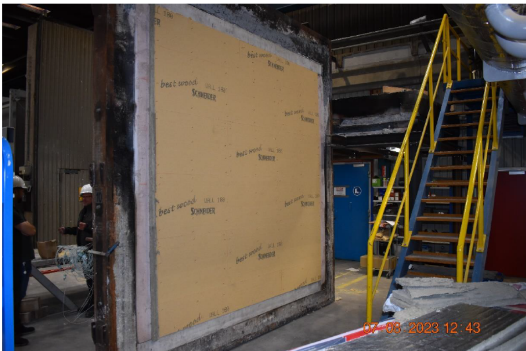
Photo No. 10 Outer layer of wood fiber board seen from exposed side
