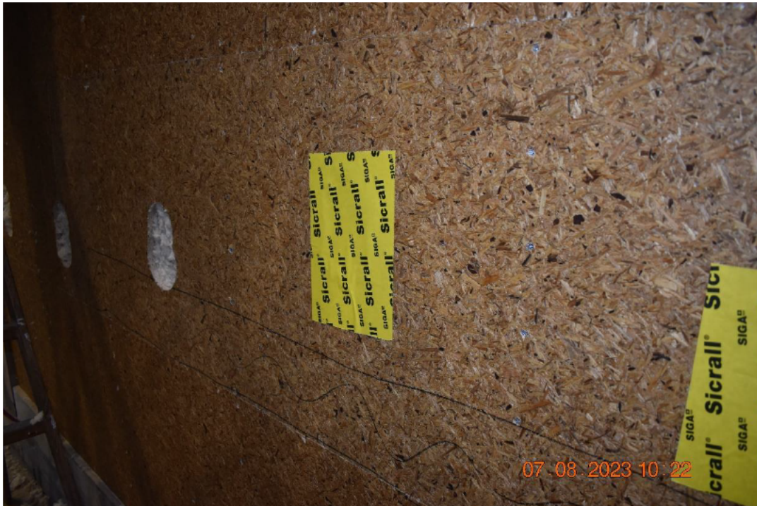
Photo No. 5 Holes are drilled and the board pieces were saved and taped back in the board layer after filling the wall with insulation.
