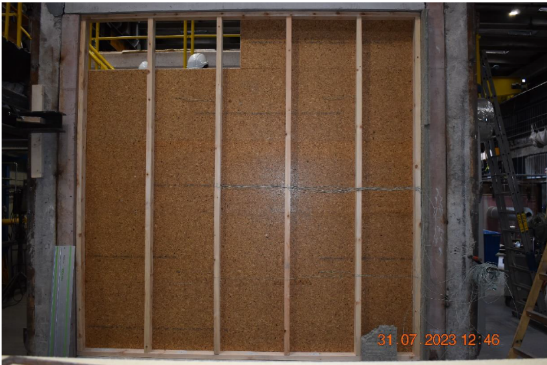
Photo No. 2 Wooden frame with first layer of boards seen from unexposed side
