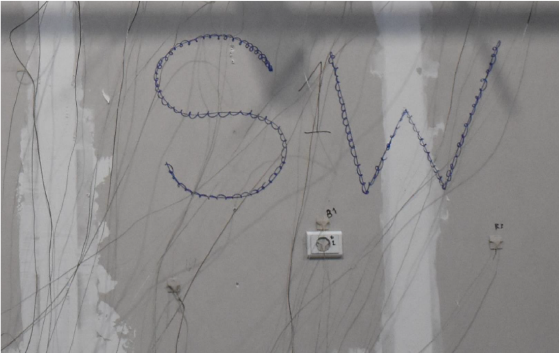
Photo No. 9 Socket before test start
