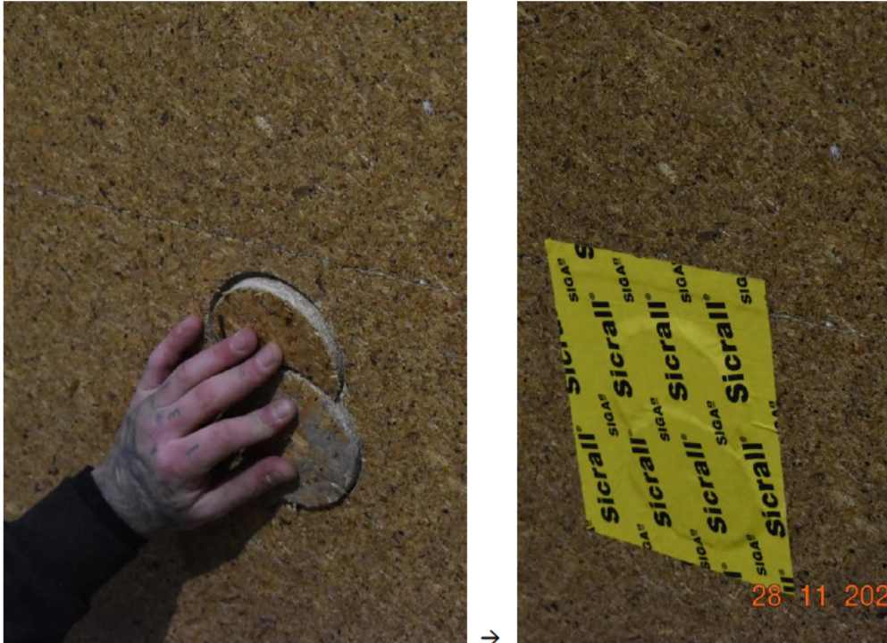
Photo No. 5 Holes for filling the construction with insulation were tape afterwards
