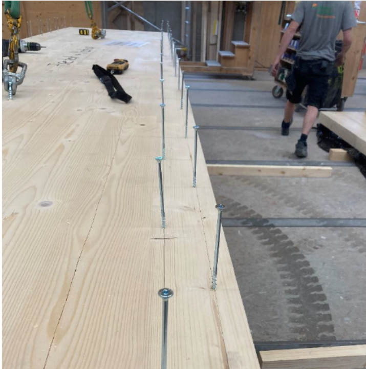
Photo No. 5 CLT-element being prepared with screws before glued to the timber beams
