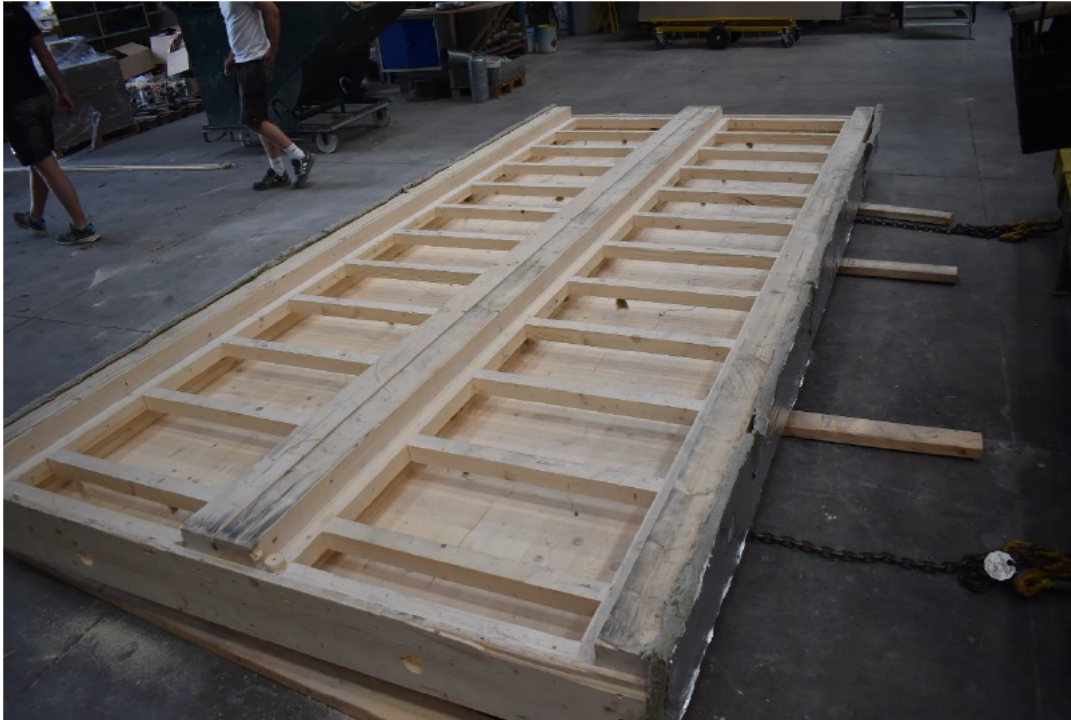
Photo No. 9 Gypsum boards and insulation is removed in order to be changed. Holes have been cut in short edge for filling of insulation
