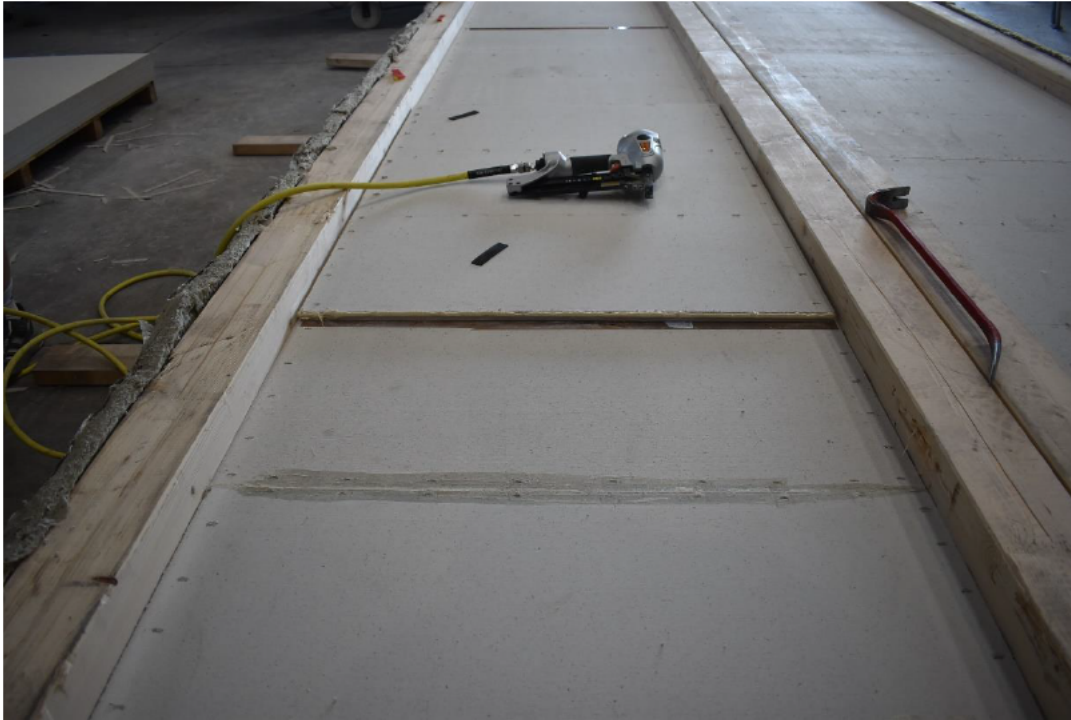
Photo No. 13 Bottom gypsum layer being mounted with glue in the gypsum joint. Plastic tape is attached behind the joints to prevent glue from reaching the top gypsum layer
