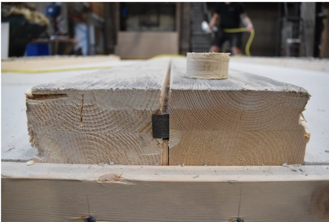
Photo No. 12 The joint between the two elements, exposed side on the on the top of the photo
