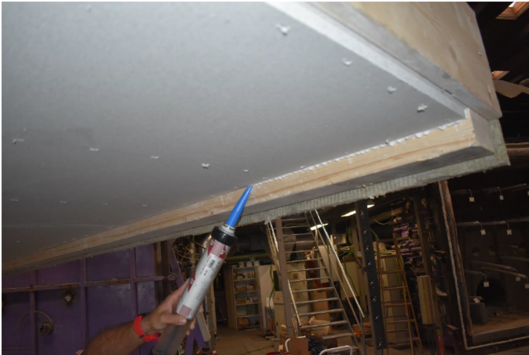
Photo No. 18 Application of sealant between the bottom layer and timber beams
