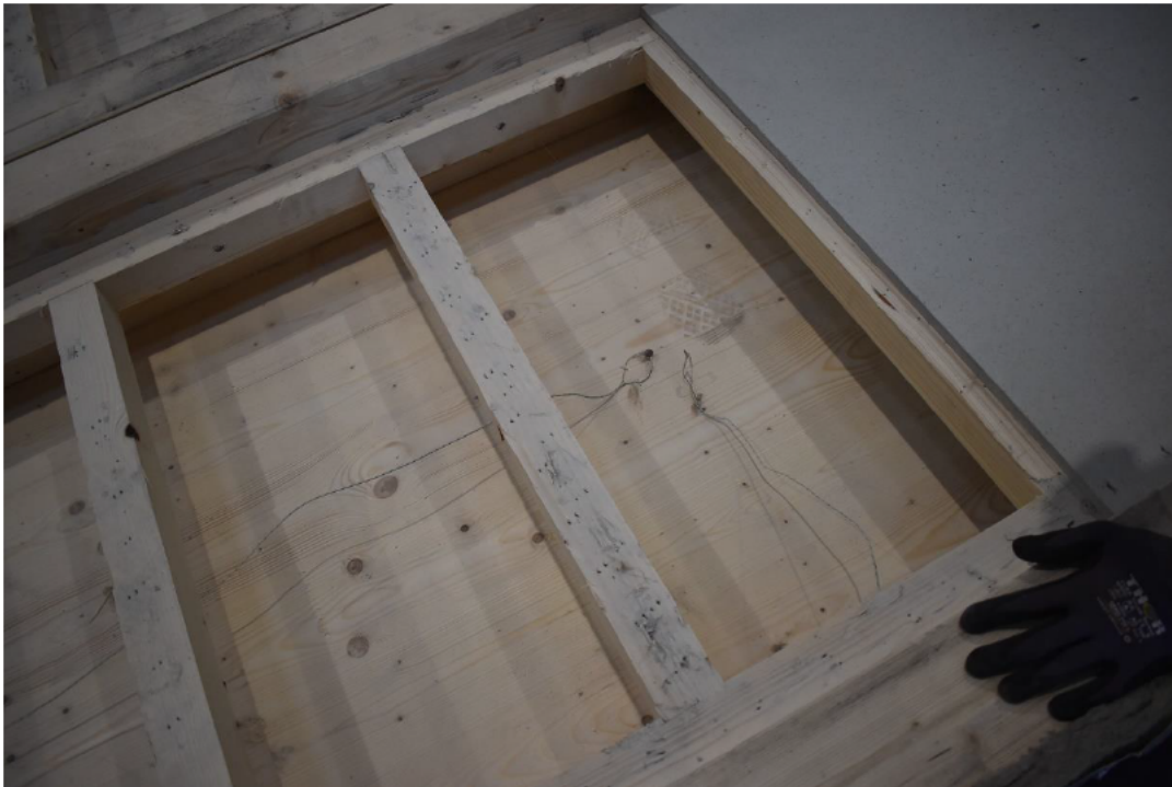
Photo No. 10 One thermocouple is mounted into the CLT-element and the other will be fixed to the gypsum board
